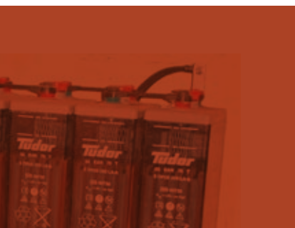
Battery Bank for PV Systems
