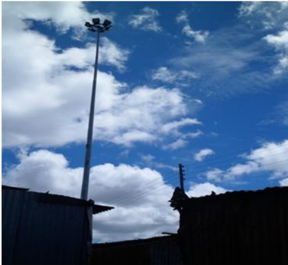
An example of a mast installed by Adopt a Light programme
