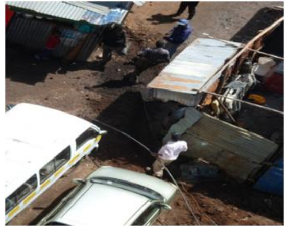
Man laying a conduit for illegal underground connection
