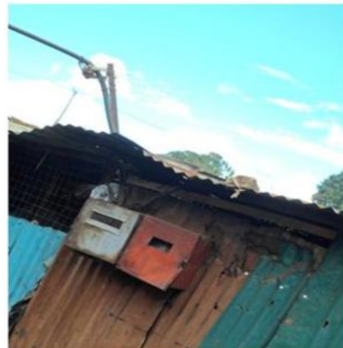
Meter boxes shown in Kibera for illegal re-
