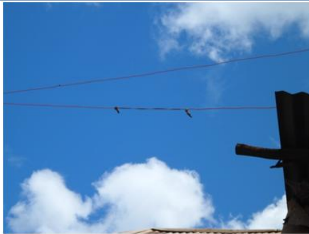
Illegal Connection of electricity in Kibera
