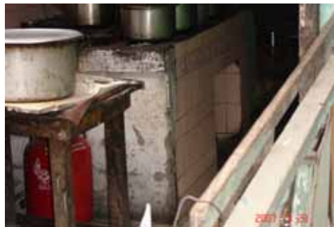
Use of domestic LPG for commercial purposes
