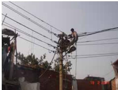
Acquiring illegal connections through hooking
