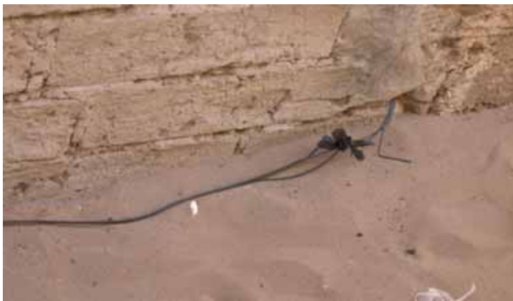
Figure 4. Example of underground illegal connections in Ben-barack
