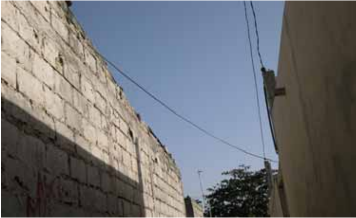
Figure 6. Example of suspended illegal connections in Ben-barack
